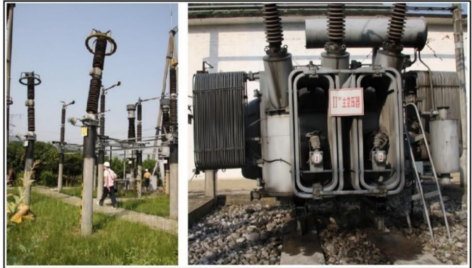
Fig 1. Destruction of power facilities in the Wenchuan earthquake.
